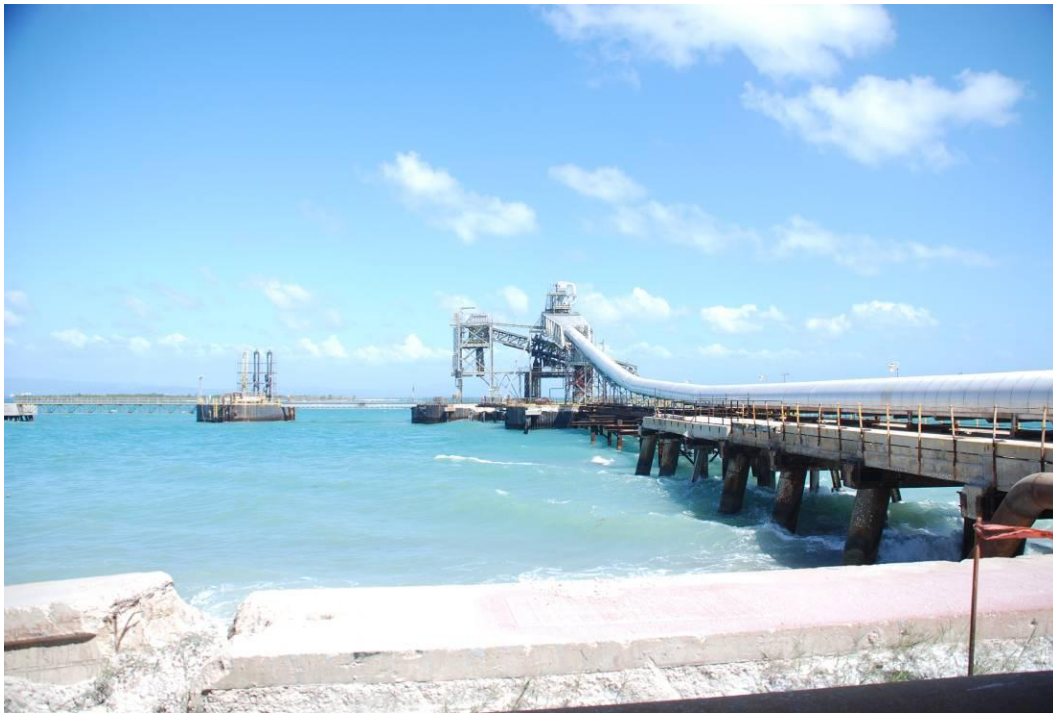
Plate 5-10: The approach road to the dock partly destroyed (middle distance). The seawall on the left was damaged by hurricane Ivan. (Photo taken 12/02/08)
