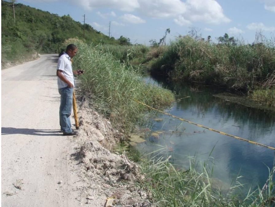
Plate 5-11: The main road from Freetown to Tarentum showing undermining from failure of the canal bank (Photo taken 08/02/08 GPS Location N 17.86784° W077.15734°)
