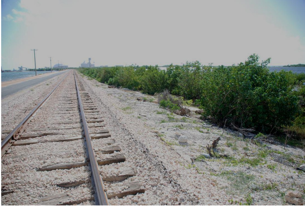
Plate 5-8: The railway approach to Rocky Point. Dean tore the lines from the track and deposited them in the area to the right where the hummocky Staghorn coral debris is located. (Photo taken: 12/02/08 GPS Location N 17.82036° W077.15578°)
