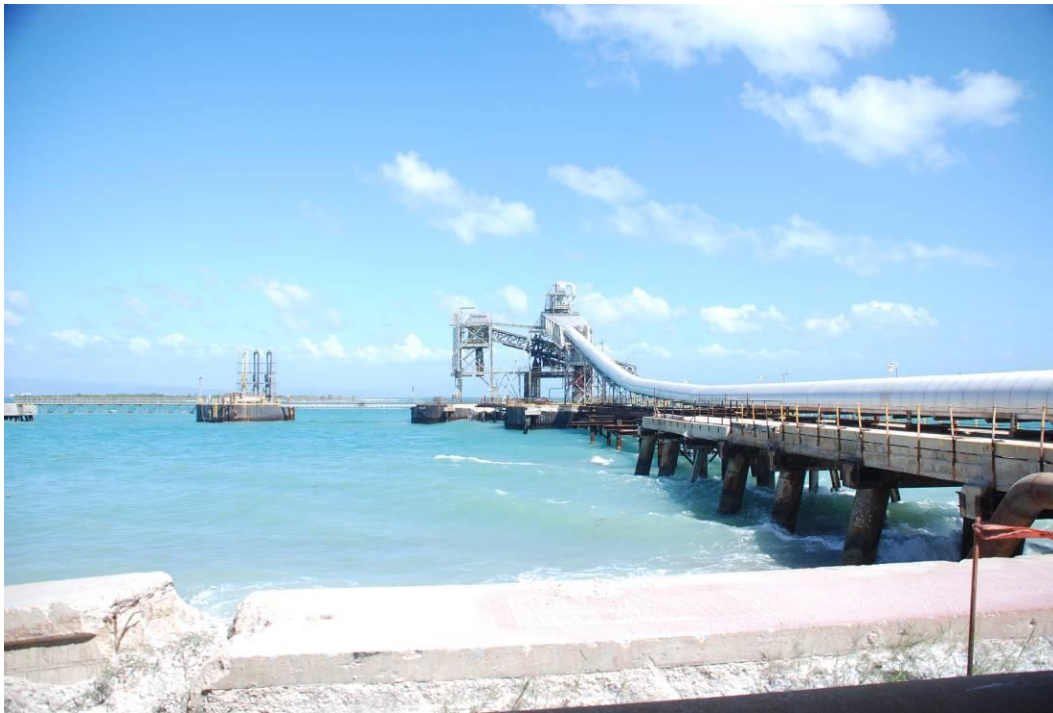
Plate 5-10: The approach road to the dock partly destroyed (middle distance). The seawall on the left was damaged by hurricane Ivan. (Photo taken 12/02/08)
