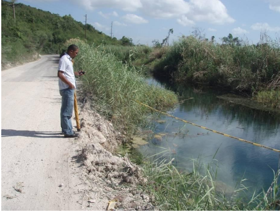
Plate 5-11: The main road from Freetown to Tarentum showing undermining from failure of the canal bank (Photo taken 08/02/08 GPS Location N 17.86784° W077.15734°)
