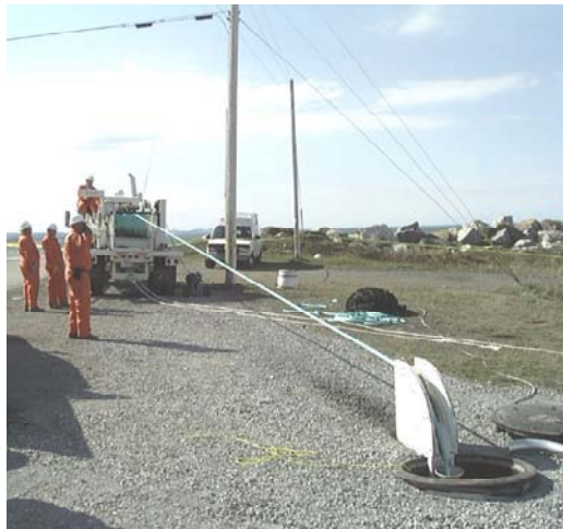
Shore-end Manhole Winch
