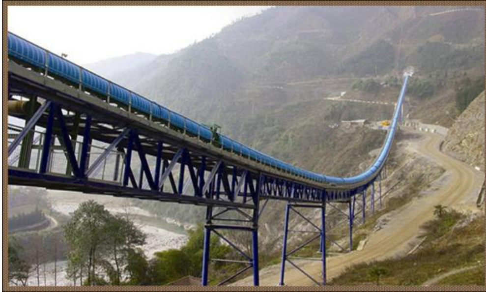
Figure 31: Photo of a typical belt conveyor
