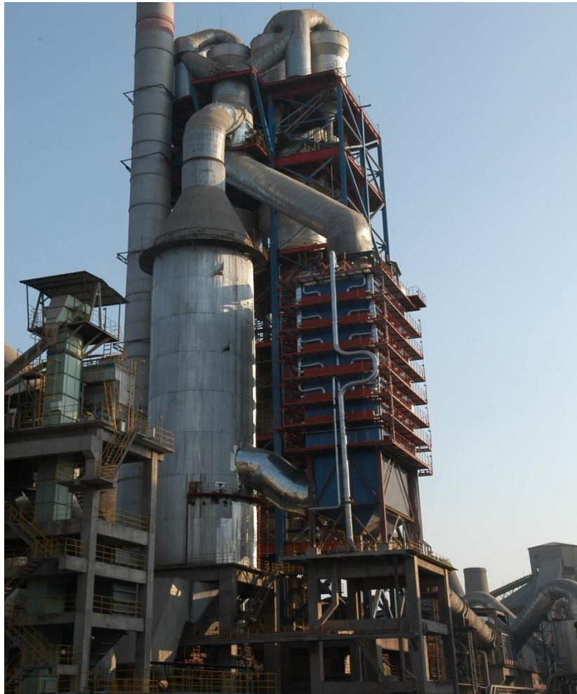
Figure 39: Picture of a typical co-generation plant
