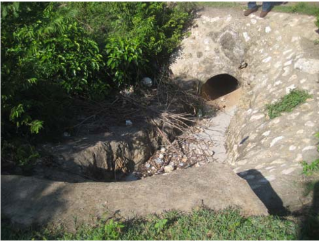
Figure 3-4. Pictures shows 36" pipe culvert 2 which channels runoff into the off site into the Mammee gully.
