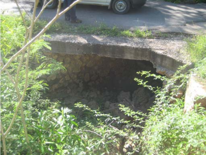
Figure 3-3. Photo of box culvert 3 under western perimeter road which channels the runoff from the Mammee gully.
