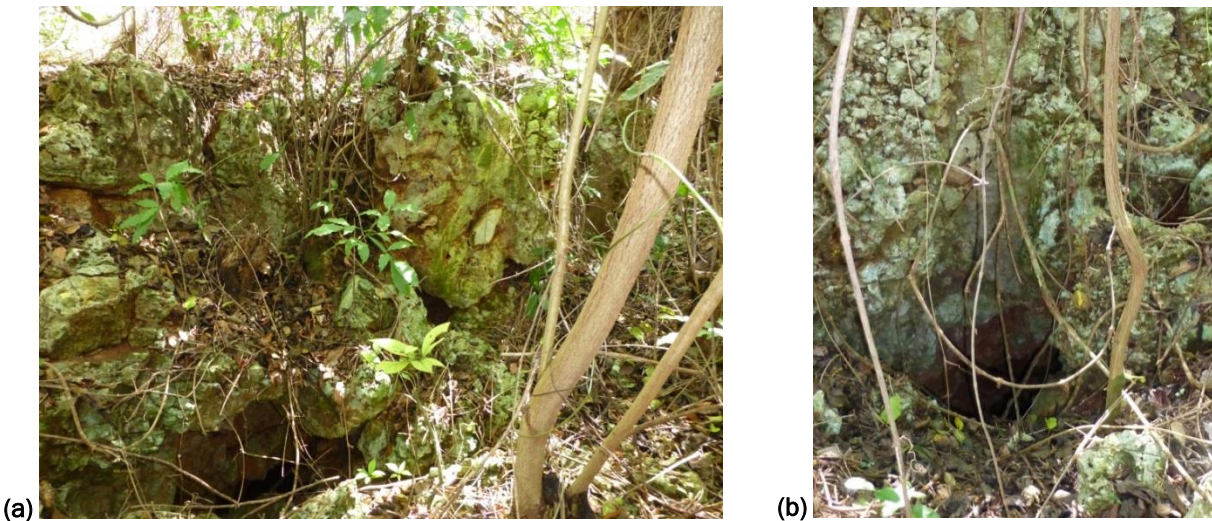
Plate 4-4 Edge of Sinkhole #1 (a) and Karst Pipe (b)
