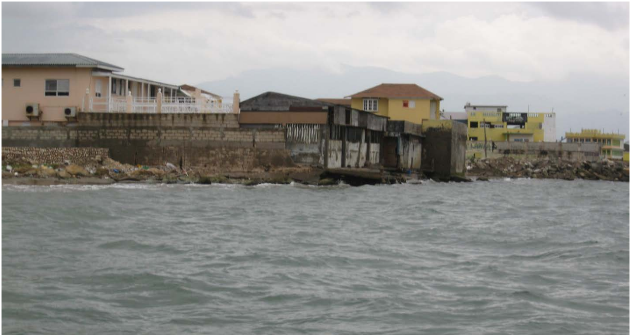
Figure 25: Severe beach erosion and structural damage along the shoreline to the west of the proposed Fort Augusta expansion area. Without mitigation, this section of the shoreline will likely experience further erosion and infrastructure damage.
