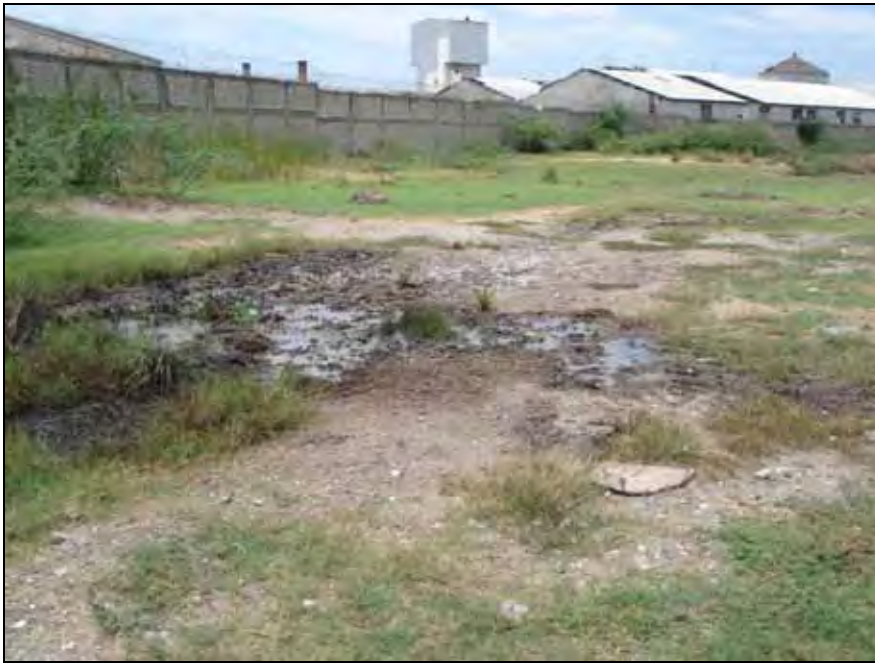
Plate 3 Example of areas of poor percolation on site
