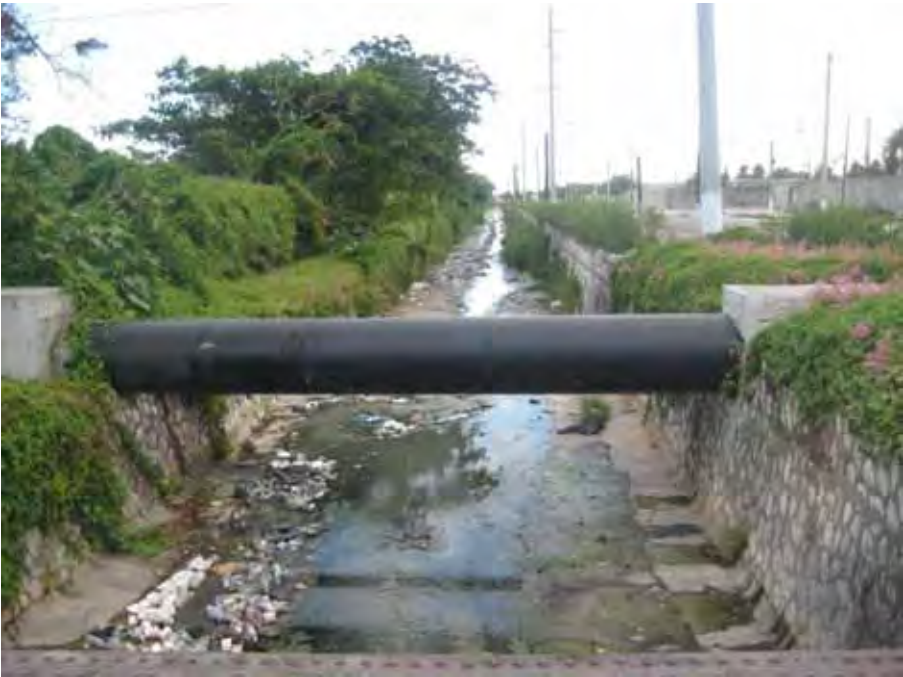
Plate 5 Picture shows concrete u-drain which borders the western boundary of the site and Industrial Terrace.
