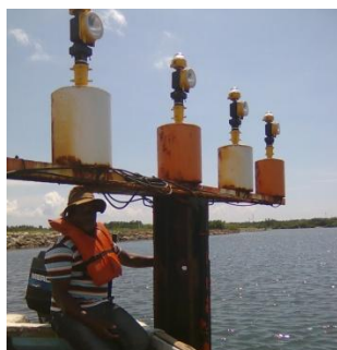
Figure 6.1.4: Existing approach light
