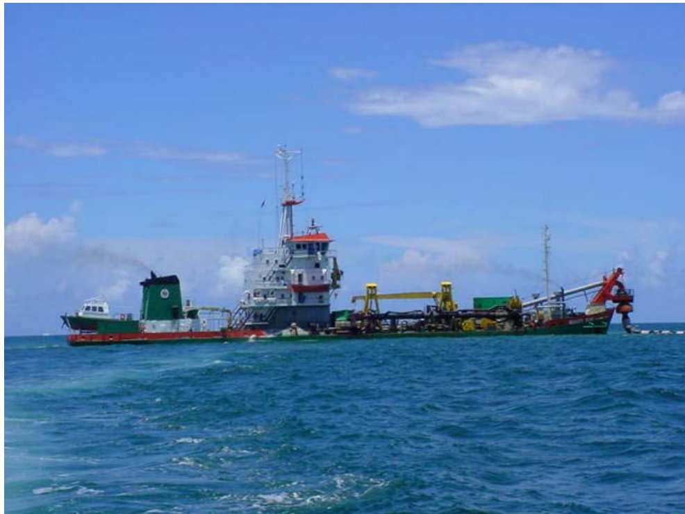
Picture 23. Quality Star trailing suction hopper dredger, belonging to ASTIMAR S. A. Company, coupled by its prow to a floating pipeline to start the sand discharge. Hopper capacity 2 400 m 3 .
