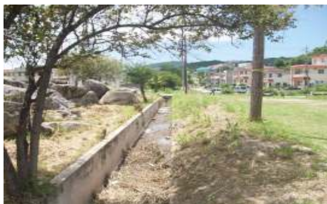
Plate 7.2: Existing drains in the Pines of Karachi
