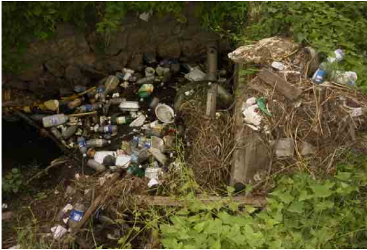
Plate 5.1.8a: General detritus, PET bottle and Styrofoam food carrier blocking the inlet to the pipe culvert beneath the Church Pen parochial road (Photography taken June 26, 2006)
