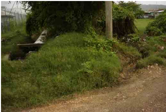
Plate 5.1.8b: Manually excavated relief drain (foreground) adjacent to the National Irrigation Commission Canal (Photograph taken June 26, 2006)
