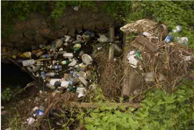
Plate 5.1.5a: General detritus, PET bottles and Styrofoam food containers blocking the inlet to the pipe culvert beneath the Church Pen parochial road ( photograph taken June 26, 2006 )
