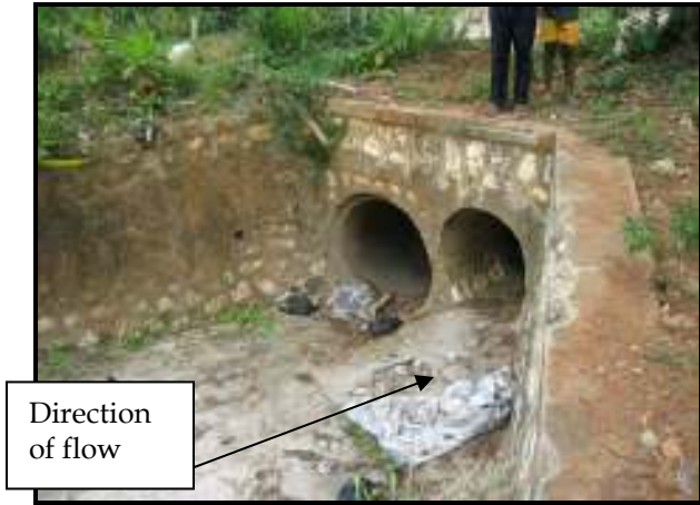
Plate 18: Culvert pipes in the single Hut Gully normally blocked during heavy rainfall
