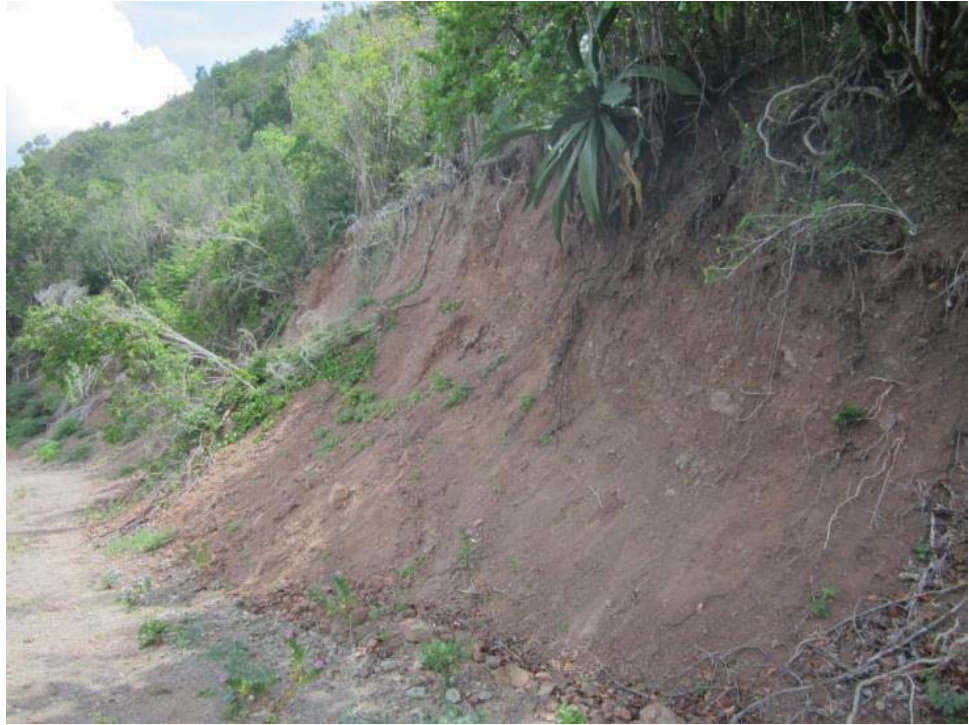
Plate 6.3 First landslide encountered during site visit (#519)
