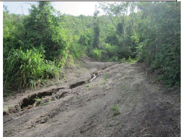
Plate 2.10 Deteriorated roadway following the passage of Tropical Storm Chantal (2013) due to lack of drainage;
