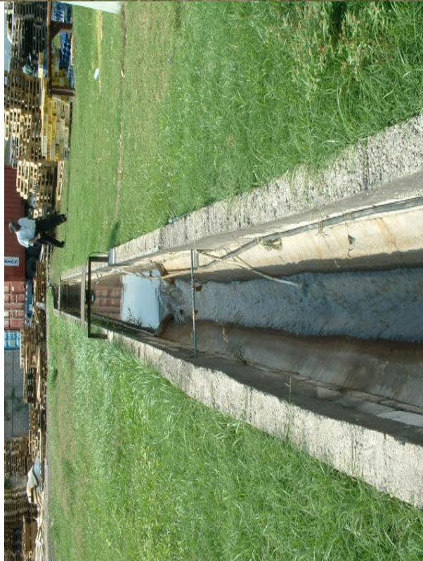
FIGURE 7-9: MONITORING STATION 1 AND ASSOCIATED DRAIN
