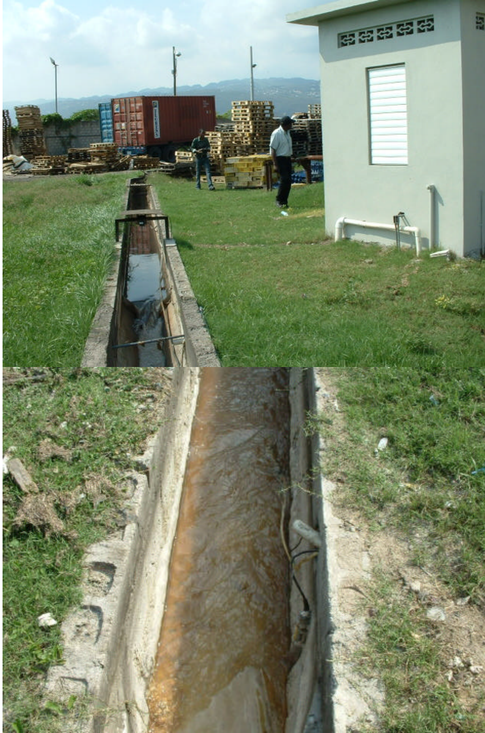
FIGURE 7-10: MONITORING STATION 2 WITH ASSOCIATED DRAIN
