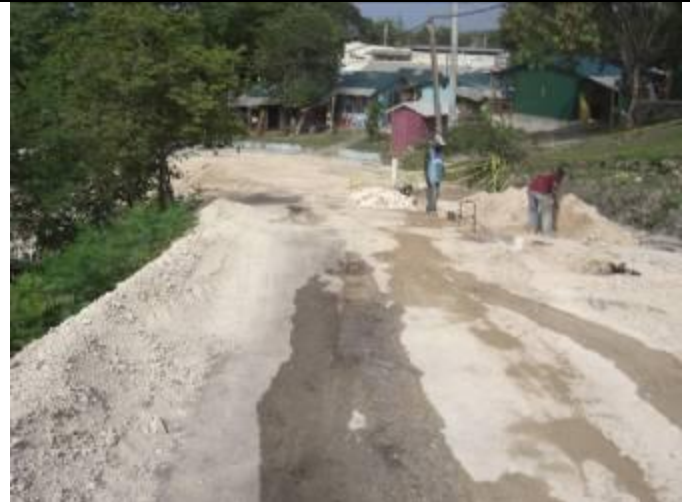
View looking North down Craft Market Road. Land route to pass on left of road. Visible works are for water utility and not associated with ALBA-1 works.
