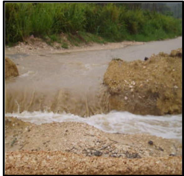
Plate 3.11: Sheet Flooding on Main Site Access Road (Chukka Cove Intersection)
