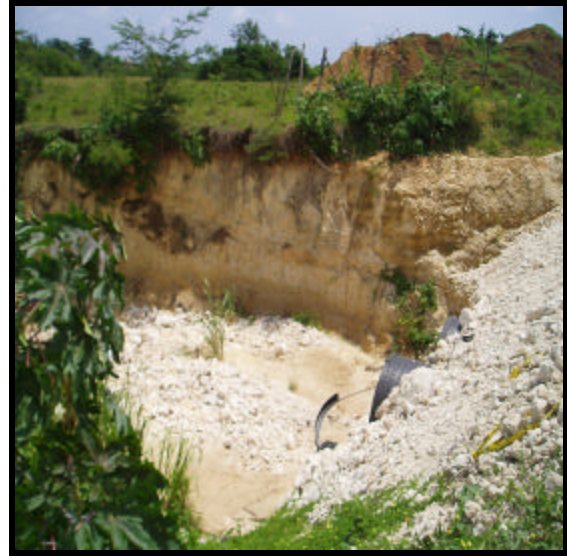
Plate 3.4: Richmond Estate Gully (Northern Exit)
