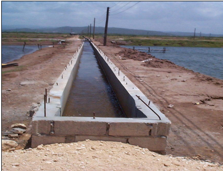
Plate 8. Concrete water supply system to shrimp ponds at CMPL.
