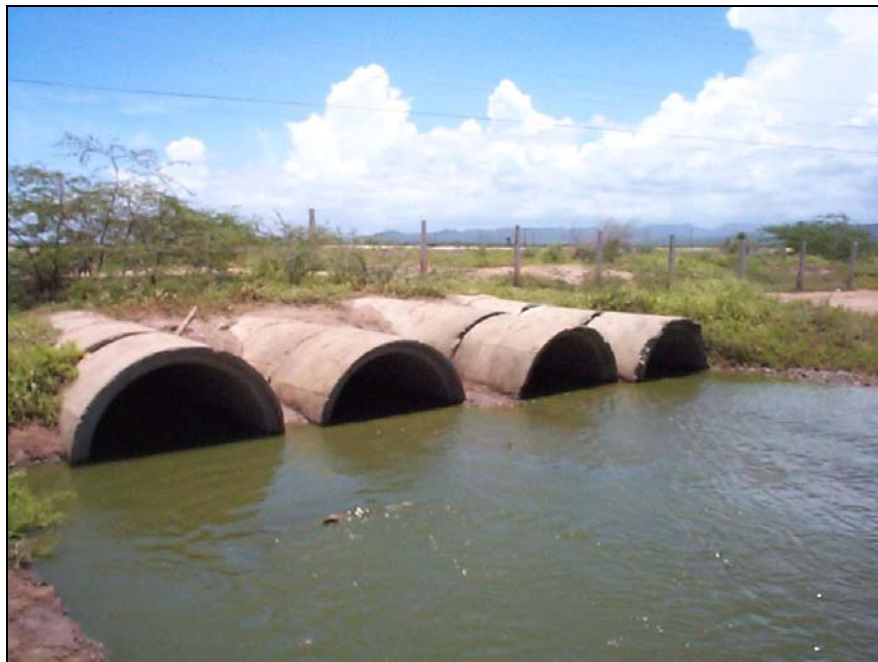
Plate 14. Concrete drainage culverts across Thompson Pen Lane. (Photo taken after clearance of culverts)
