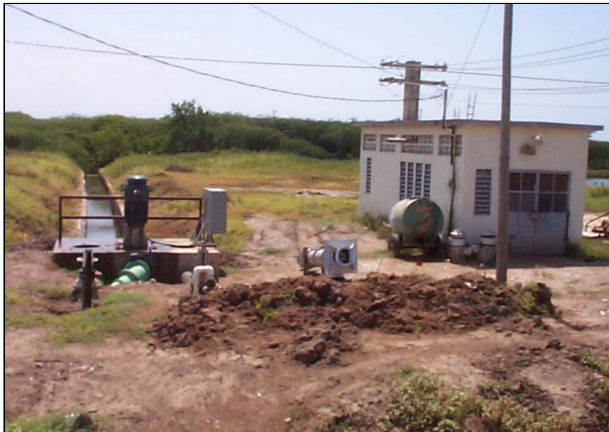
Plate 3. Existing pumping station extracting water from Frasers Gully, Brampton, St. Catherine.
