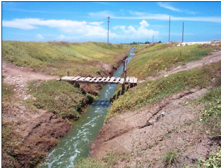
Plate 12. Erosion of outer sides of drain embankments at CMPL.
