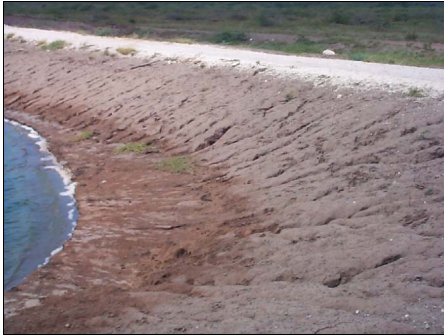
Plate 11. Erosion of inner sides of pond embankment at CMPL.
