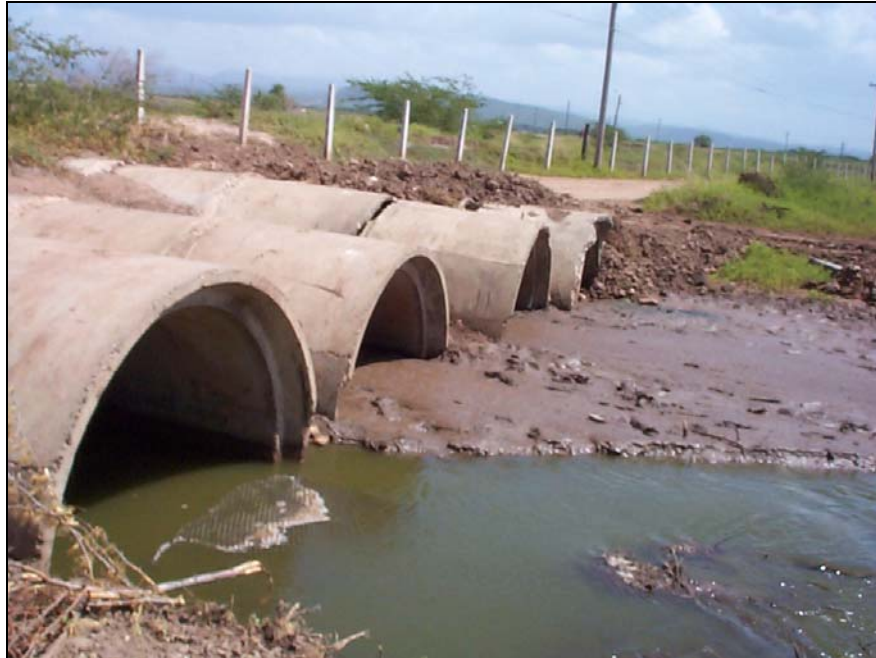
Plate 15. Sediment deposits at culverts across Thompson Pen Lane.
