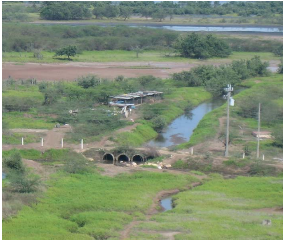
Photo 2 Culverts in the watercourse to the south crossing the eastern parochial Road
