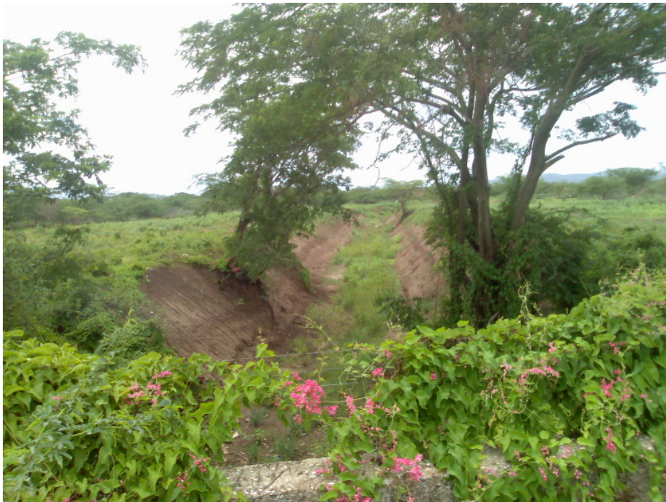
FIGURE 4 - NEWLY CONSTRUCTED EARTH DRAIN THAT FLOWS TOWARD FRASERS GULLY (PHOTO LOOKING EAST)
