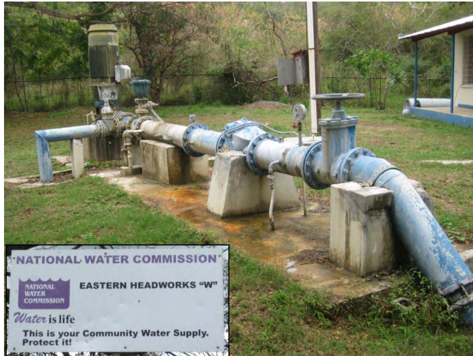
Plate 4.24 - Photo showing WQ2 – NWC Eastern Headworks 'W' well
