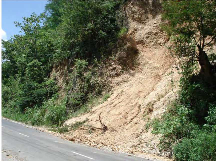
Plate 4.18 - Land slip on the southern edge of the fault zone exposed along the main road at the northern entrance to the Bog Walk Gorge (Walderston formation). This location is within the same Bog Walk Fault zone as will be traversed by the proposed highway.
