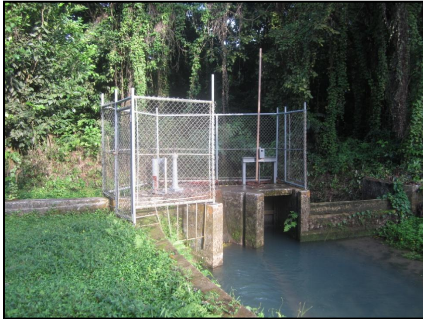
Plate 4-10 Sluce gate implemented within the channel of Roaring River
