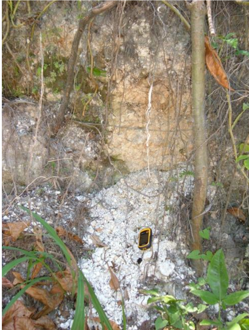
Plate 4-12 - Small scale slope failures observed within the Montpelier Formation. These are indicative of the soft rubble nature of this unit (yellow & black GPS unit in photo for scale)
