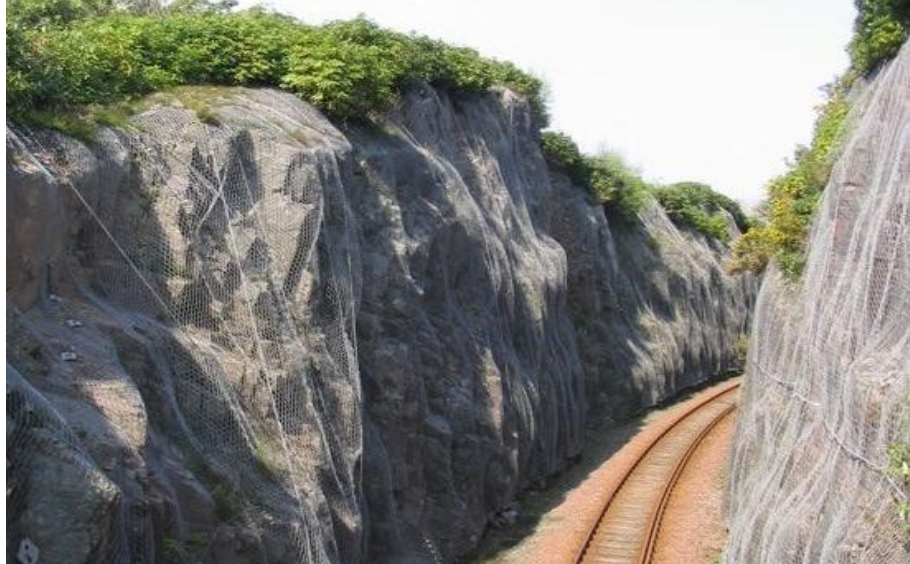
Plate 9-9 - Rockfall netting used to protect trains from falling rocks
