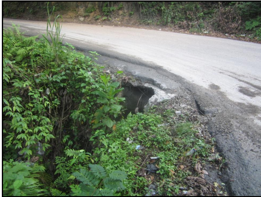
Plate 4-6 Exposed culvert pipe under existing roadway.
