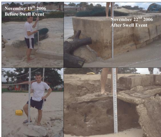
Figure 6. Localized erosion at the Negril river groyne and southern end of Long Bay.
