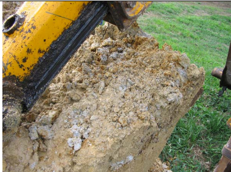
Figure A.16: Pit 7 Mottled yellow-brown and grey clay excavated at base of pit below perched watertables
