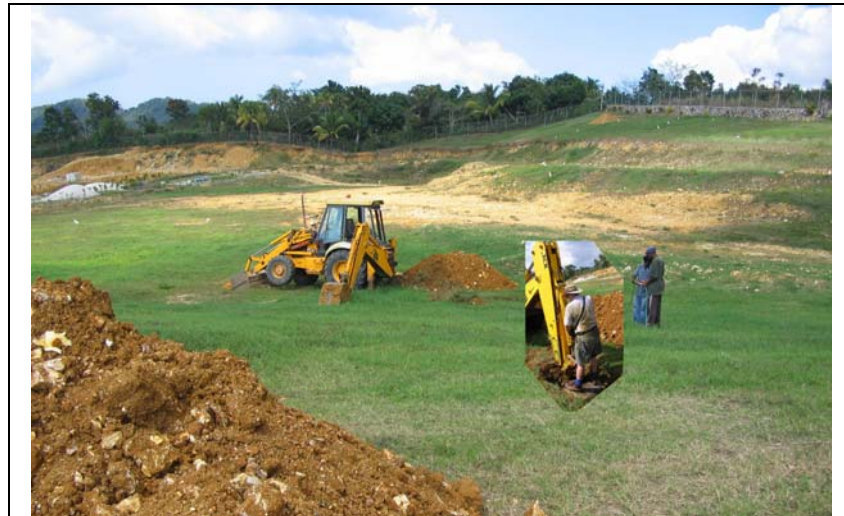
Figure A.8: Pit 4 location in major drainage area; soils noticeably damper
