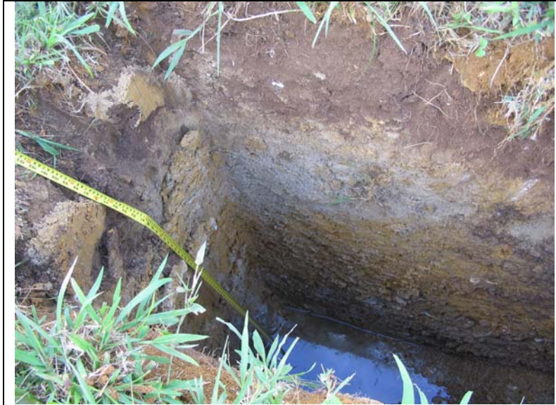
Figure A.15: Pit 7 Groundwater inflow continues as perched watertables struck within next 0.5 m; water level rises
