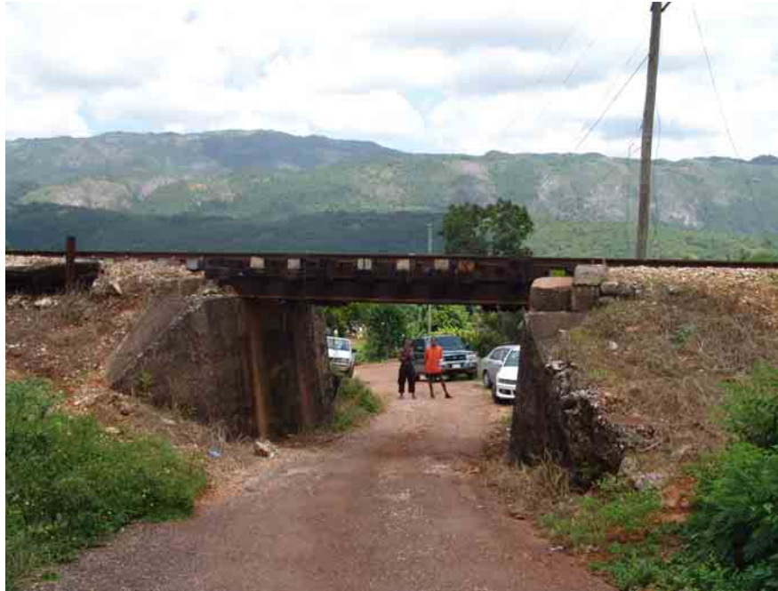
PLATE 1-2: SMALL BRIDGE NEAR BROADLEAF WHICH NEEDS TO AND WILL BE ENLARGED AND UPGRADED
