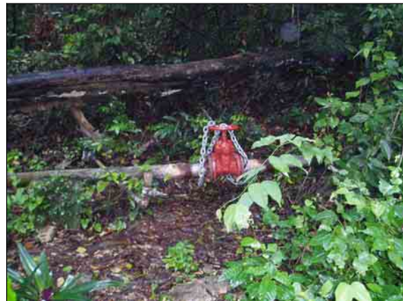
7/b Pipeline and valve.
