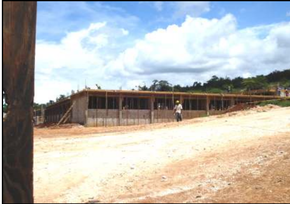
Plate 21: The new high school being constructed adjacent to the Bluefields All – Age School
