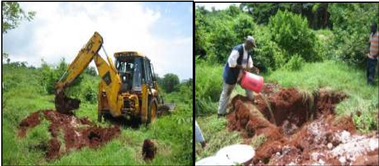
Plate 1: Excavation of test pit for conducting percolation test with the assistance of a backhoe.
