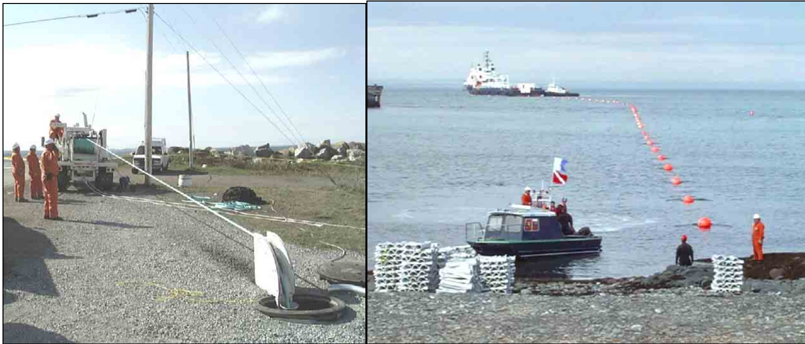
FIGURE 1-19: ILLUSTRATION OF INSTALLATION WITH A WINCH ON THE SHORE; BUOYED CABLE ON THE RIGHT
