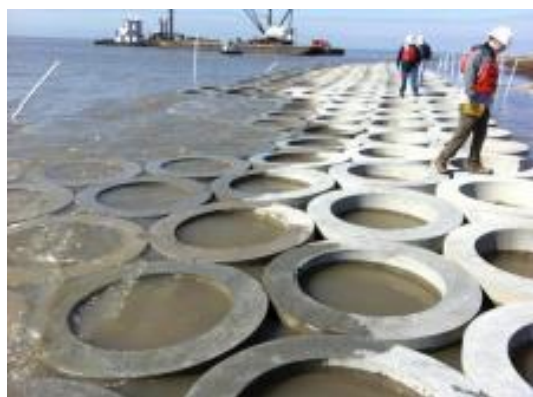
Figure D2 Example of use of shoreline protection structure which has been adapted to provide wider natural benefits. Picture shows installation of the concrete pods.
