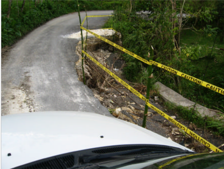
Figure 14 - Broken roadway in the Great River WMU
