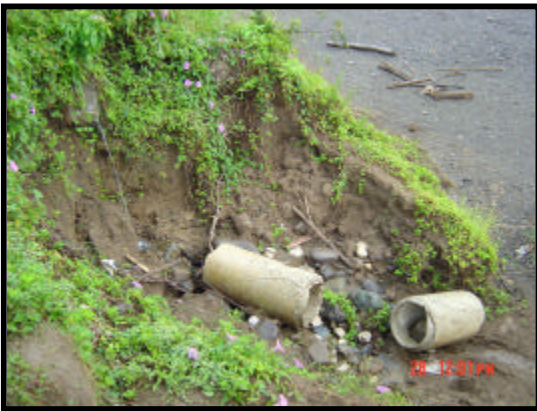
Figure 5. Destruction of physical infrastructure induced by bank erosion at the Berridale Rafters Rest.
