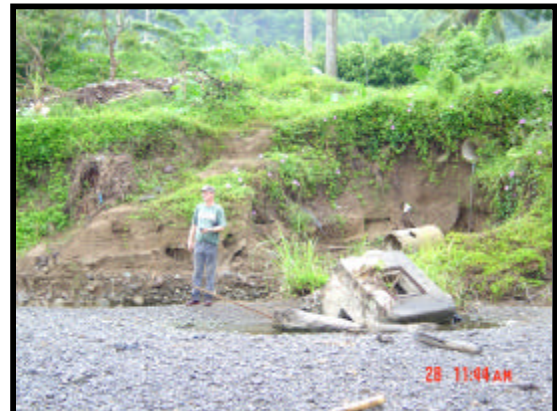
Figure 6. Destruction of physical infrastructure induced by bank erosion at the Berridale Rafters Rest.
