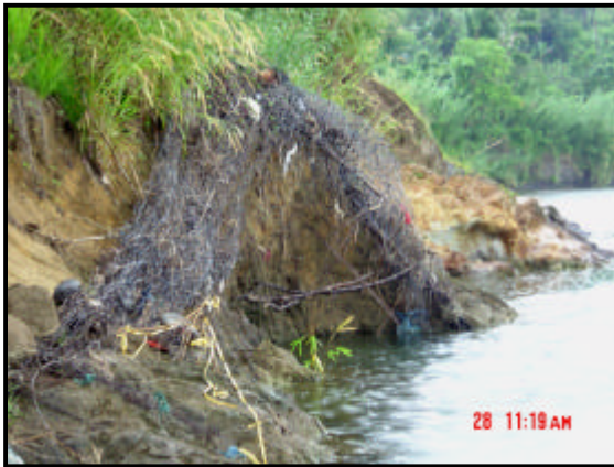
Figure 11. Ruptured gabions induced by massive bank collapse on the right bank of the Rio Grande River at Berridale.
