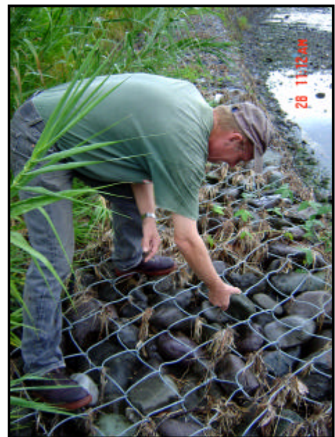
Figure 10. Dr. David Miller demonstrates the poorly constructed nature of gabion baskets at Berridale. Here, mesh size > cobble and boulder material
