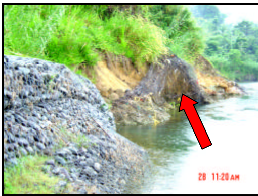
Figure 9. Gabion baskets recently constructed, along the right bank of the Rio Grande River. To the immediate right, ruptured gabions are exposed by an erosion scar.
