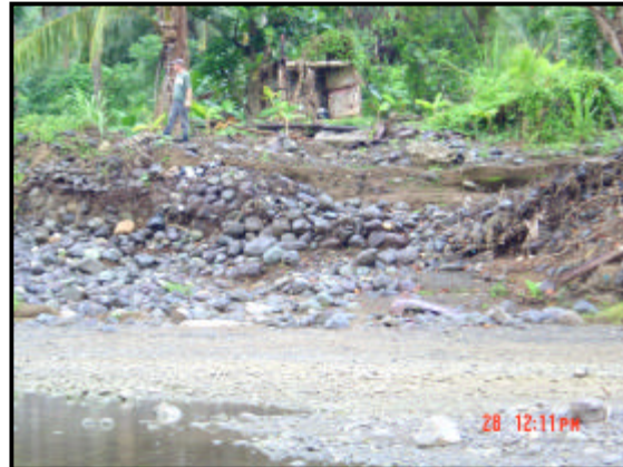
Figure 12. Damaged gabions around the sand mining operation at Berridale induced by stockpiling and loading of sand and gravel.
