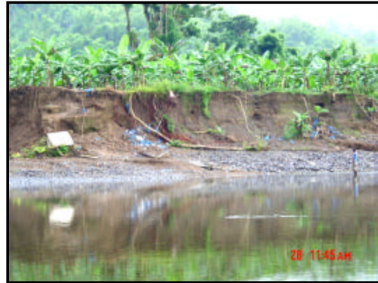
Figure 4. Extensive bank erosion on relatively straight reaches of the Rio Grande River at Berridale.
