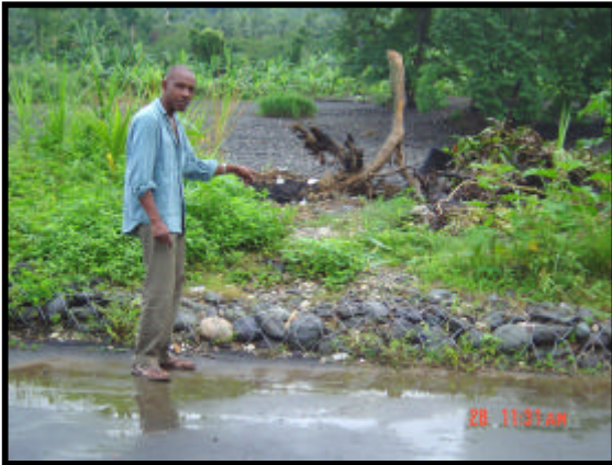
Figure 1b. Berridale resident, Mr. Miller, indicates where the gabion baskets were breached during the Hurricane Ivan flooding.
